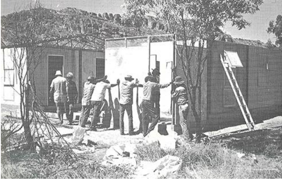
Local residents at Looma erecting their housing as part of the Commission's self-help scheme, 1978
